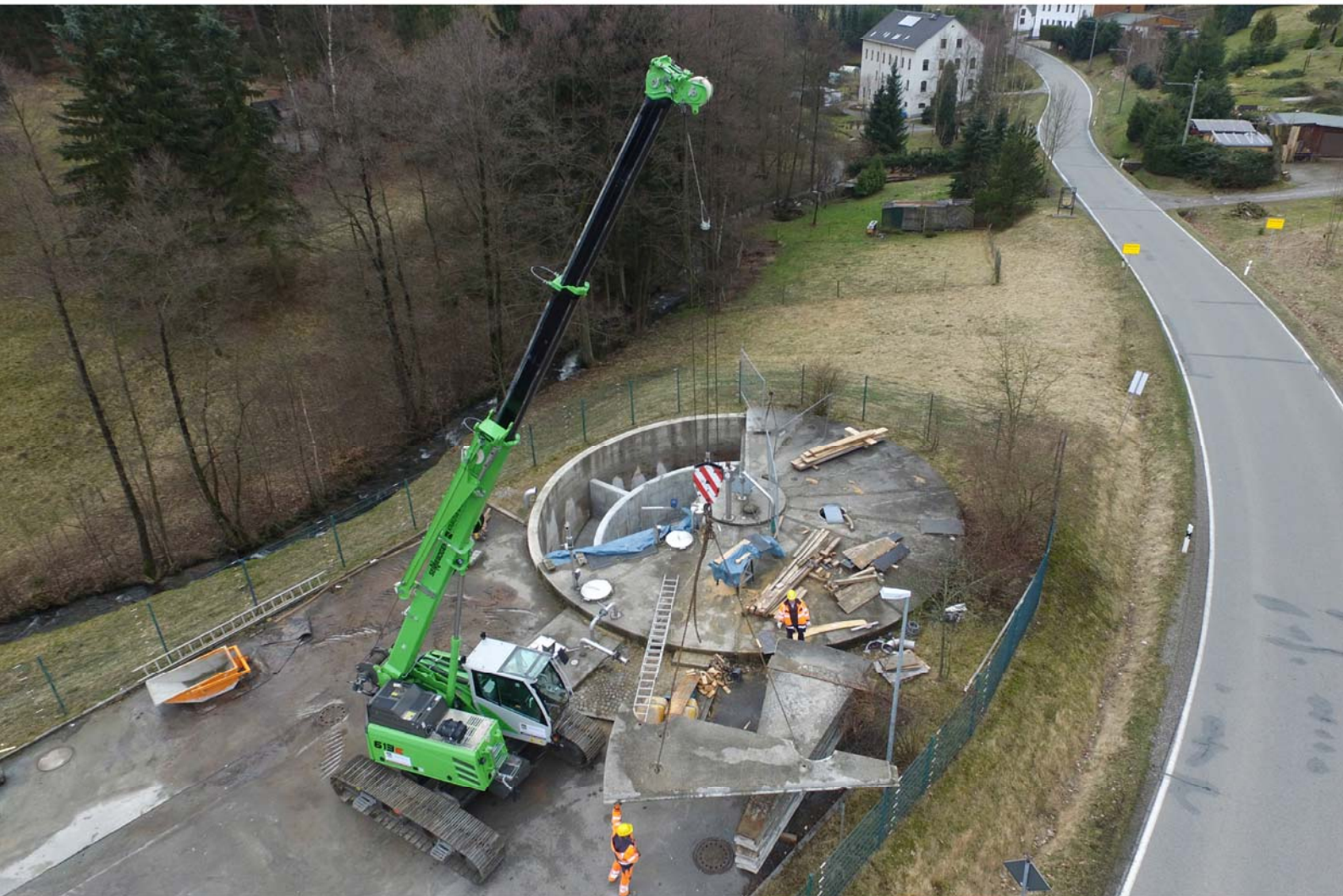
The SENNEBOGEN 613 E crawler crane moves and lifts loads on the construction site of a temporary sewage treatment plant in Germany.
